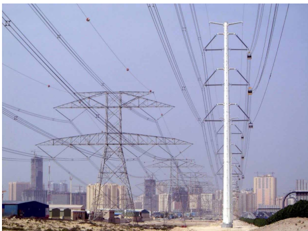
Figure 6: 400 kV compact line (right) parallel to a 400 kV conventional line (left), DEWA, UAE
